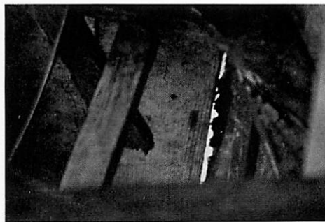
Daylight shows through her bottom planking.
