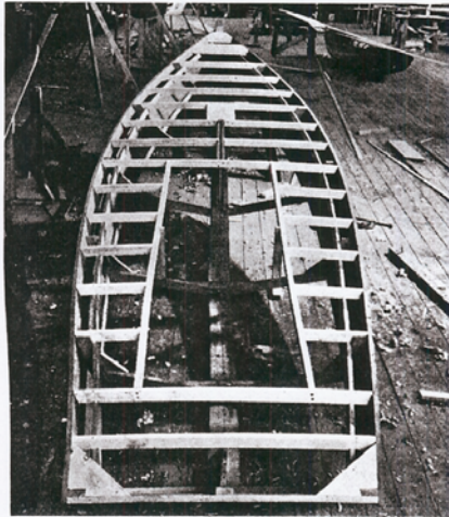
27—Deckbeams in place. Note reinforcing at stem for jib stay, mast and at stern
